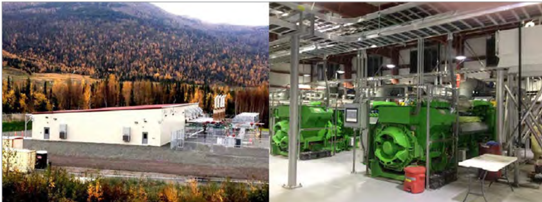
(U) Figure 5. (left) Methane Power Plant
