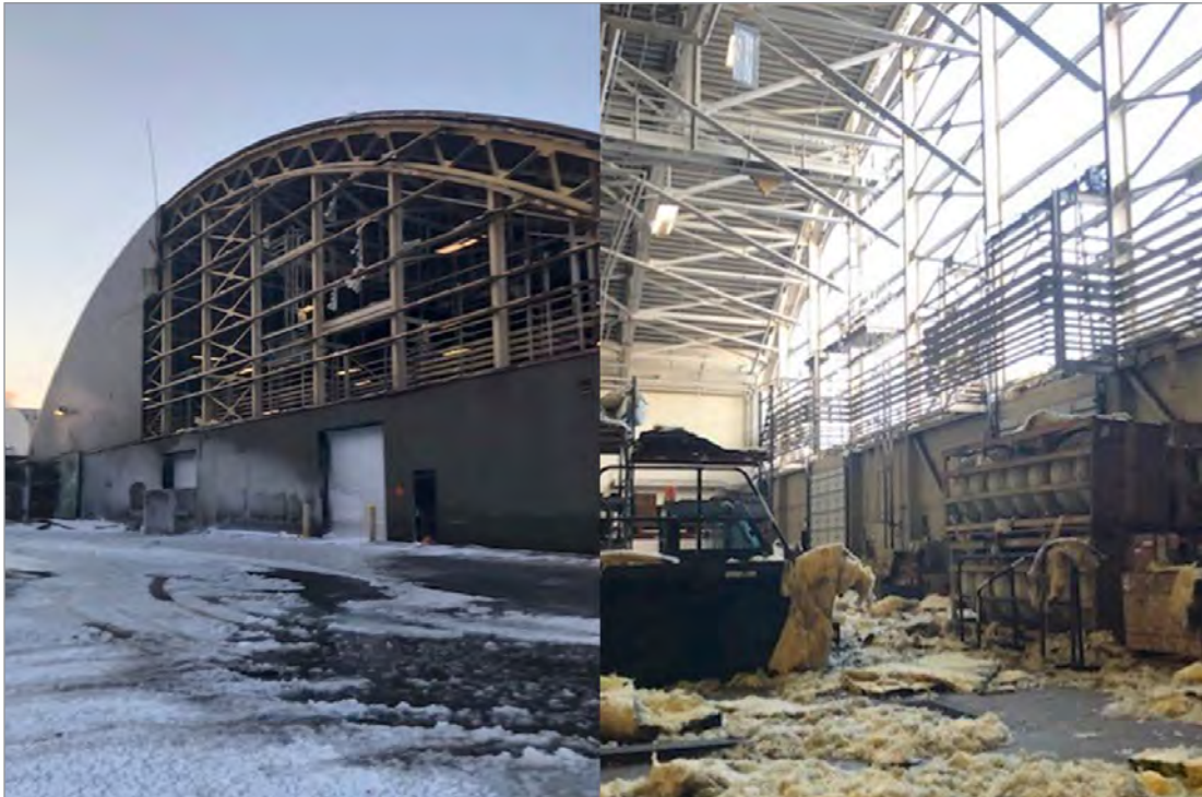
(U) Figure 2. (Left) Storm Damage to Hangar 7 (Exterior), Eareckson Air Station, Alaska (U) Figure 3. (Right) Storm Damage to Hangar 7 (Interior), Eareckson Air Station, Alaska (U) Source: 611th Civil Engineering Squadron.
