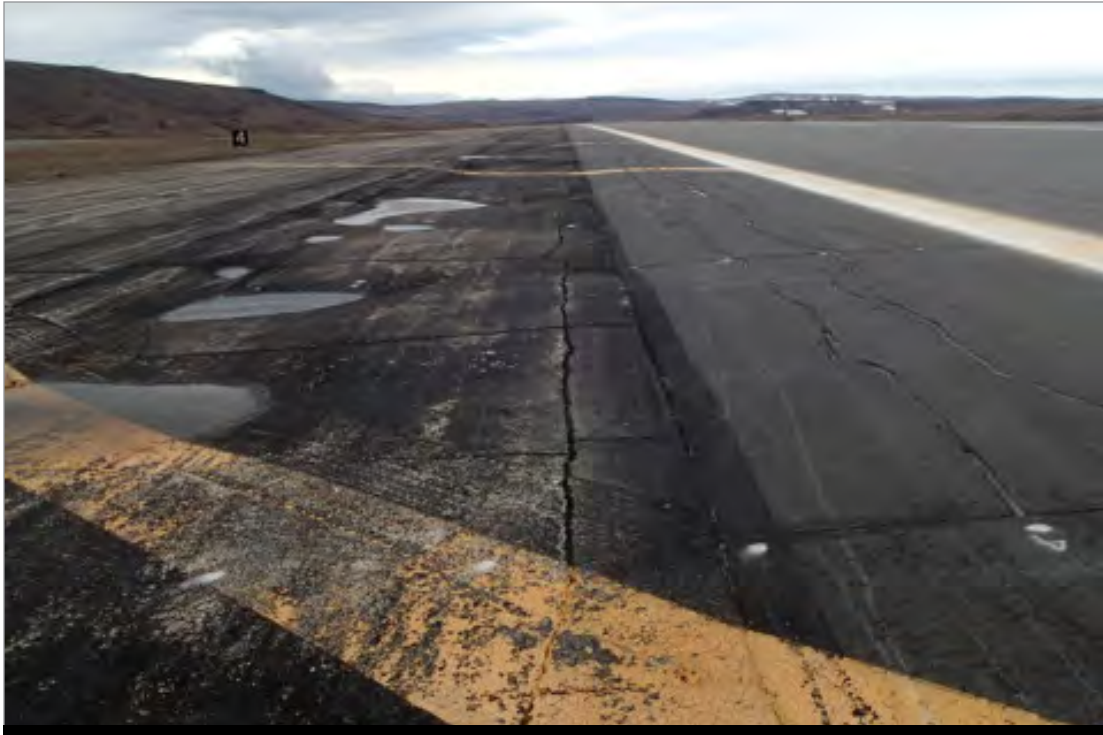
(U) Figure 7. Cracks and Depressions on Runway and Shoulder Caused by Water Thawing and Refreezing, Thule AB, Greenland (U) Source: The DoD OIG.
